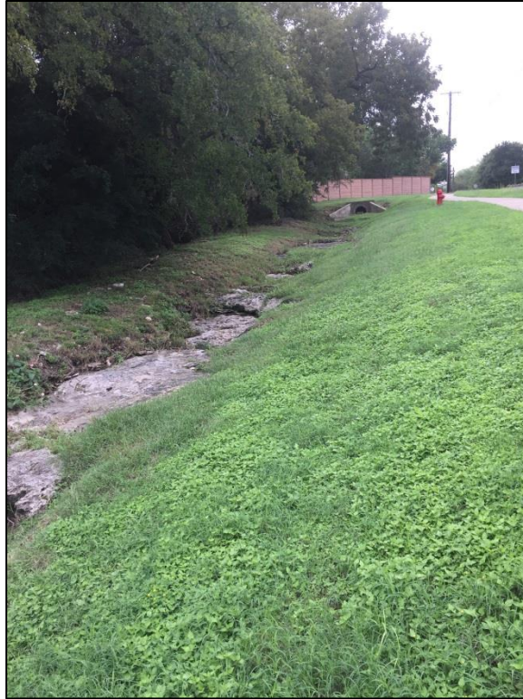
Figure 8. Erosion in Great Oaks Drive ROW, showing exposed bedrock.
