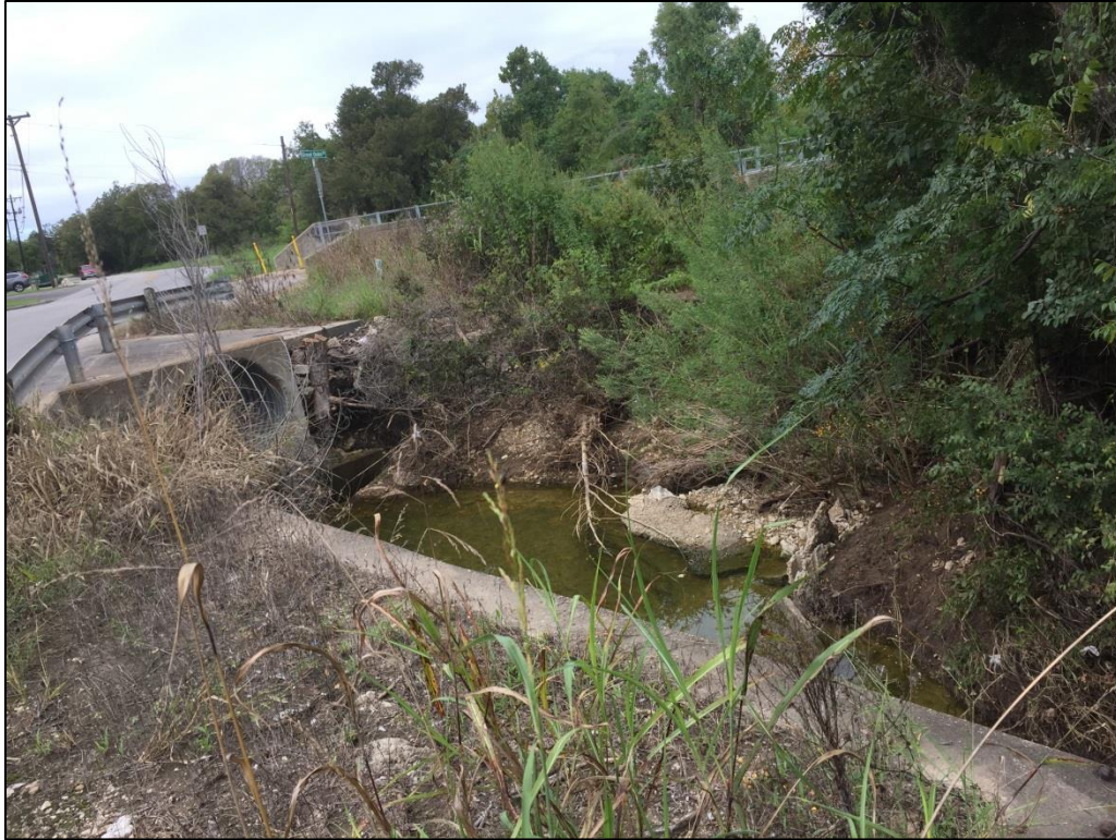
Figure 12. Erosion below culvert beneath Hairy Man Road at Great Oaks Bridge.
