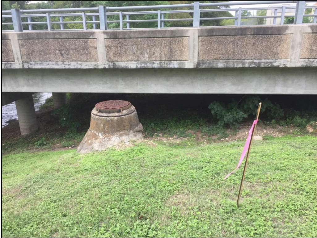
Figure 16. Sewage line in ROW on east side of Great Oaks Drive Bridge.
