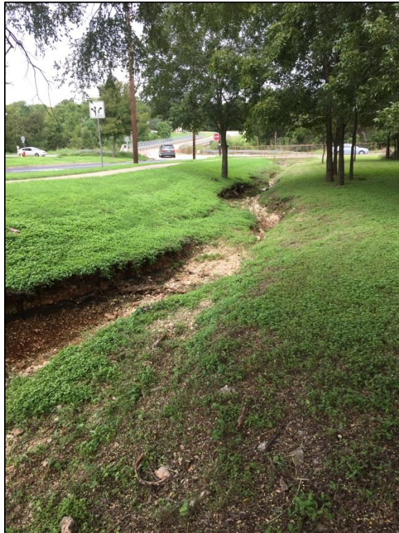
Figure 9. Erosional gully on east side of Great Oaks Drive.
