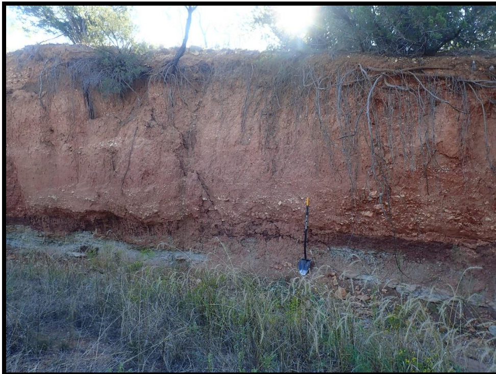
Figure 6. Eroded drainage channel of unnamed tributary of McKenzie Creek, facing east
