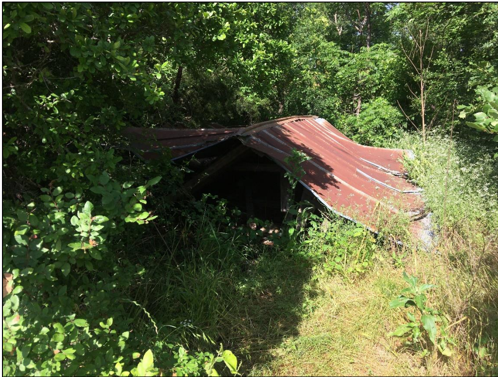
Photo 31. Collapsed structure on western side of Hartrick Bluff Road, outside of roadway ROW. View to the west.
