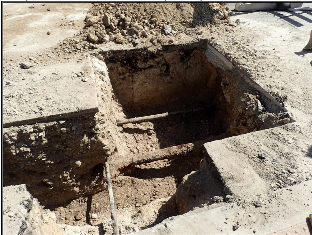
Figure 14. Exposed old gas ML and other utility lines at western terminus of ML 1.
