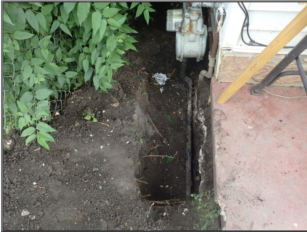
Figure 19. LSET 1 at connection with house meter, facing north.
