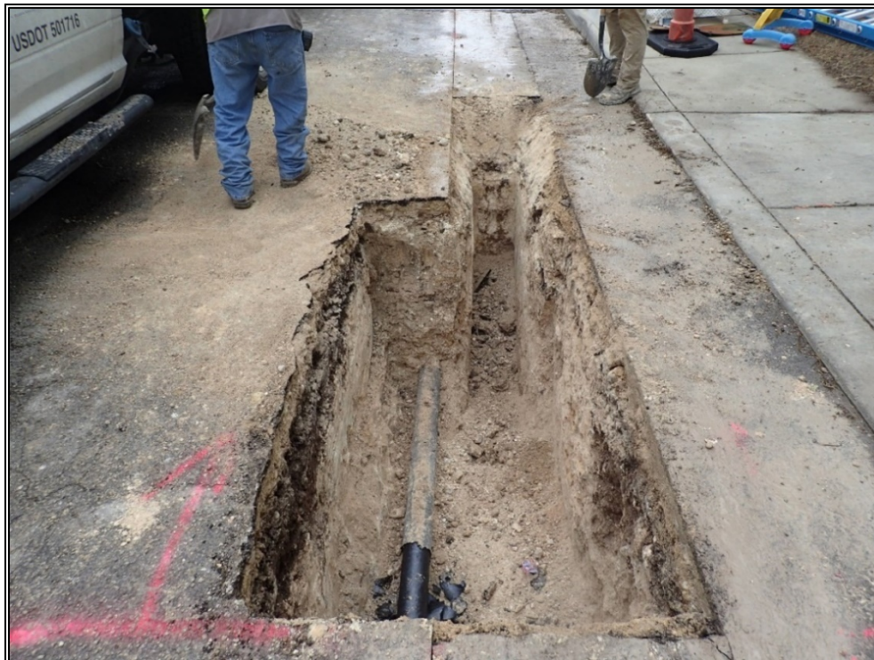
Figure 16. ML 1 at the eastern terminus showing excavated trench for new ML (right) and existing old gas ML (left).
