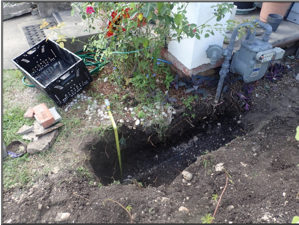
Figure 21. LSET 3 at meter connection with house, facing northwest.
