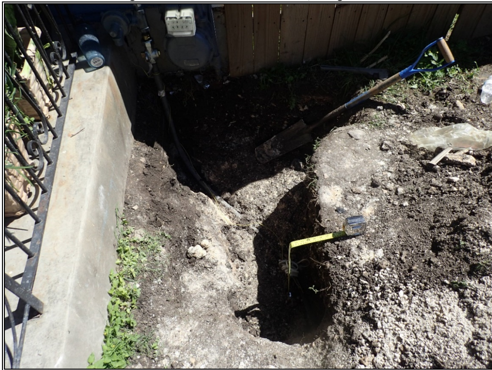
Figure 24. LSET 4 at connection with house meter, facing south.
