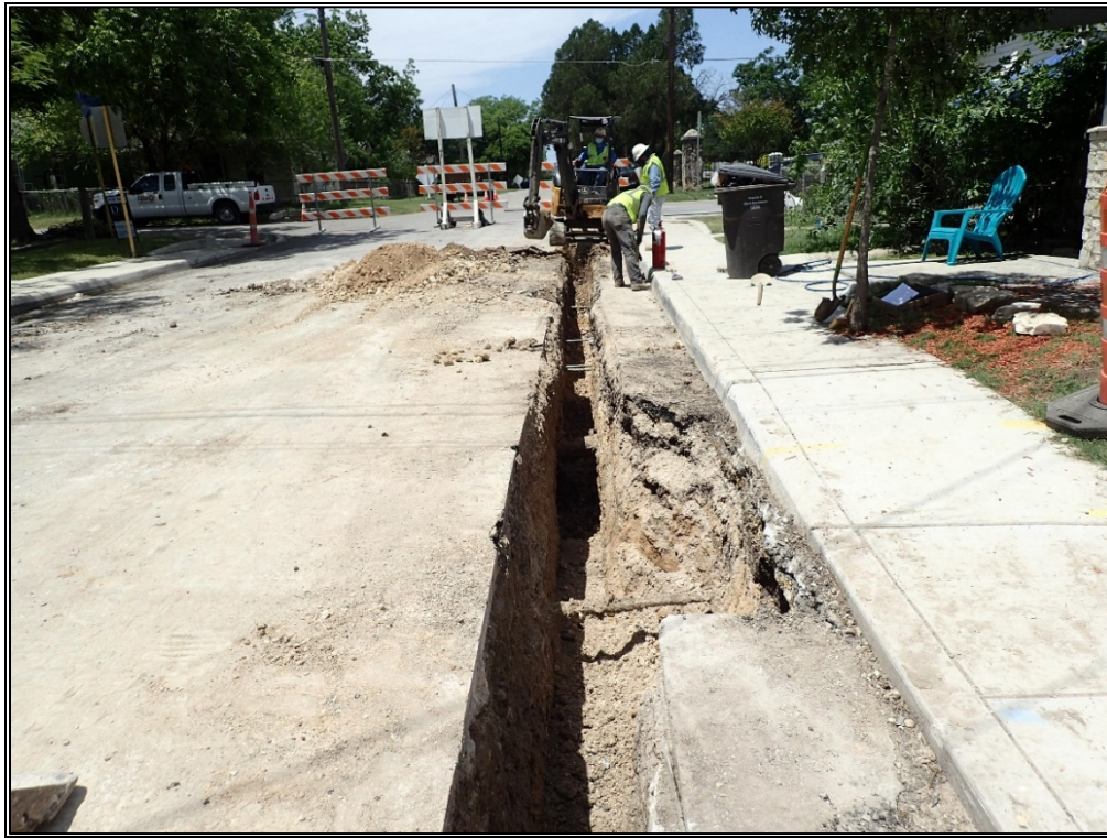
Figure 13. Overview of ML 1 from near the midpoint, facing west towards St. James Road.
