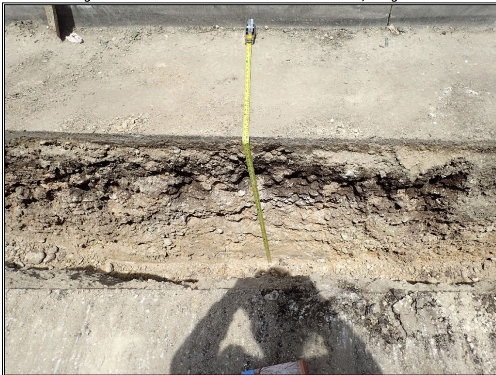
Figure 18. Close-up of typical ML 1 profile, photo is of a portion of the north wall of the trench.
