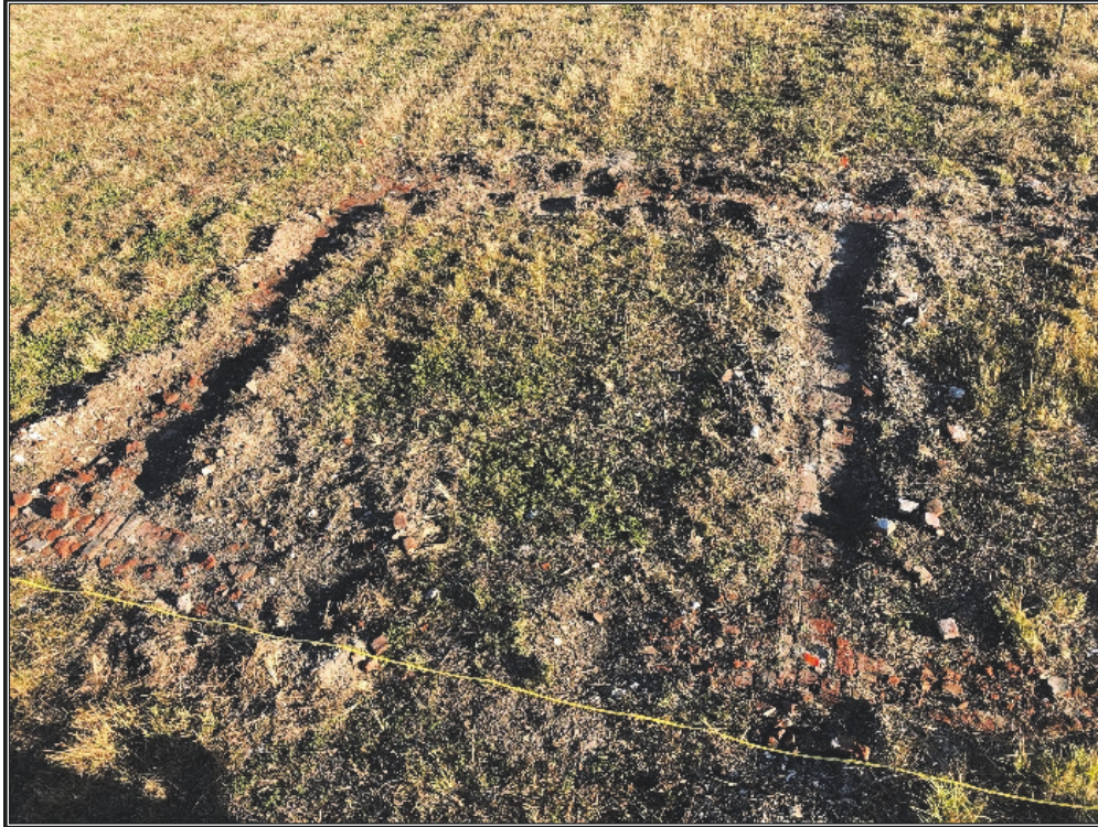
Figure 5.28a. Photo of exposed rectangular brick foundation (from atop ladder) – East side, - looking south; cross wall is shown in photo.
