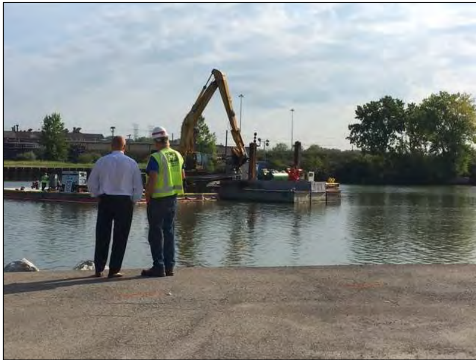
Figure 1. Contaminated sediment remediation in the lower River Raisin (credit: U.S. Environmental Protection Agency).
