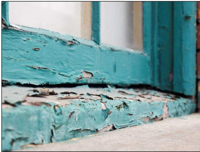
Figure 1. Deteriorated lead-based paint is one of the leading causes of lead poisoning in Detroit children (credit: Center for Urban Studies).
