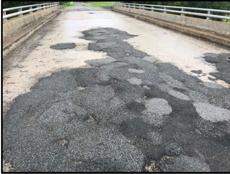
Figure 1.2. Deteriorated concrete bridge deck crossing Interstate 40 near Alma, AR (by Casey Jones).
