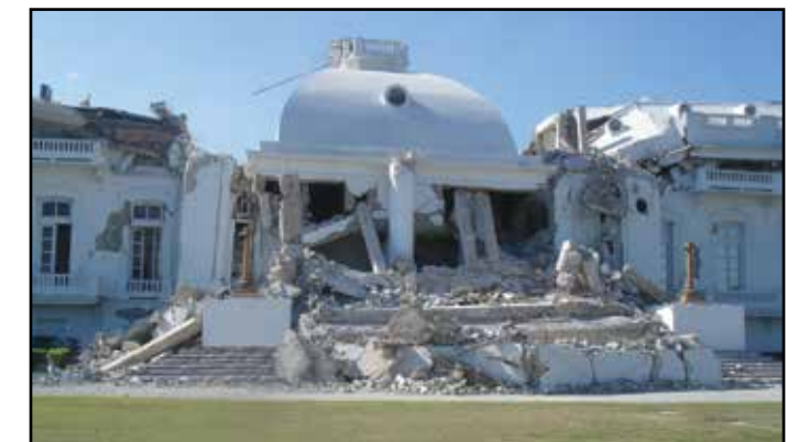
Researchers tested soil stiffness and layering on the grounds of the Presidential Palace, which was near a large area that suffered widespread destruction.
