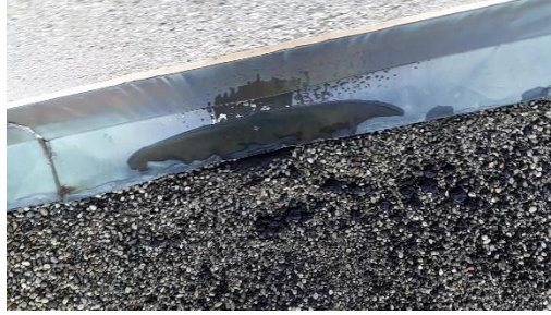
Fig. 4.12: Example of a Flashing Defect
