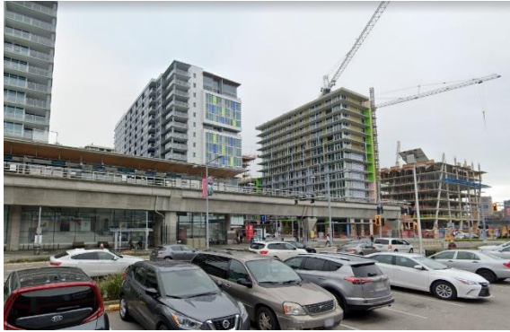
Figure 4.10 New high rise condominium developments under construction in Richmond Centre Source: Google Maps Street View
