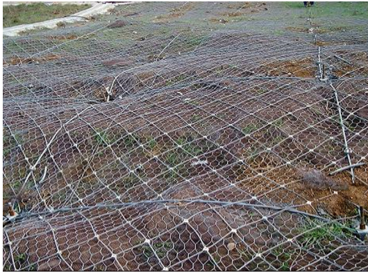
Fig. 1. Flexible membrane anchored to the ground.
