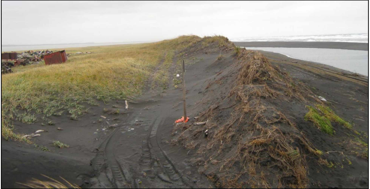
Figure 43. Photograph showing remnants of an overwash and flooding event at the access road from the beach to the solid waste disposal site, which can be seen to the left. October 2018.
