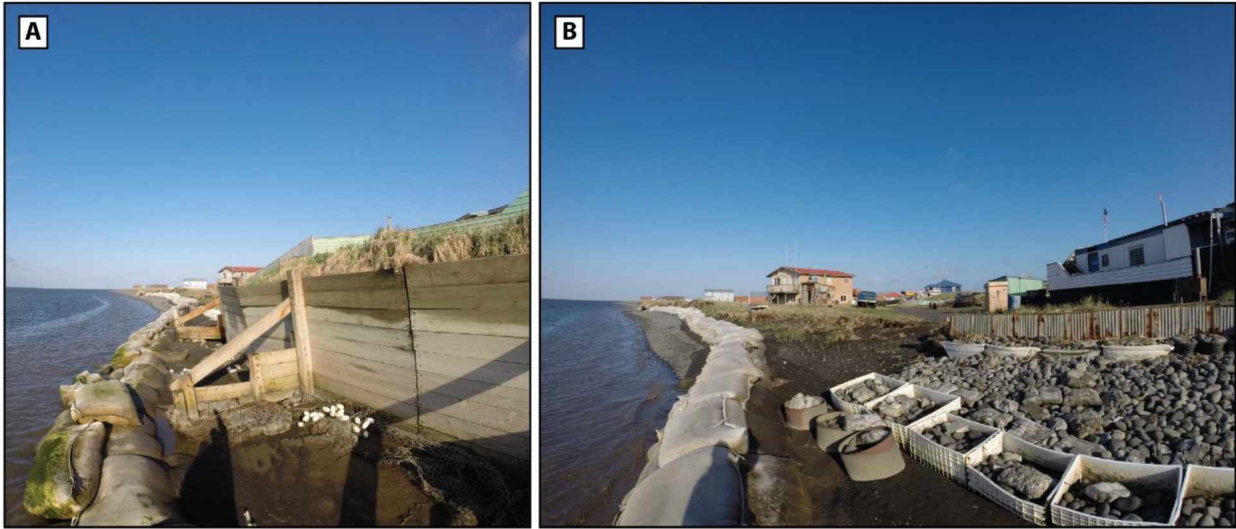
Figure 41. Seawall and sediment containers in place along the lagoon coastline of the community. A) the seawall and gabions, the geotextile containers can be seen on the left, and B) the geotextile containers fronting the community to the west of the seawall. May 2019.
