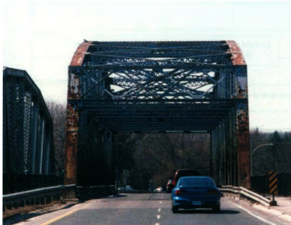
Figure 1-2: Corrosion in Salt Spray Zone of East Brough's Bridge (London, ON) (Jelinek 2002)
