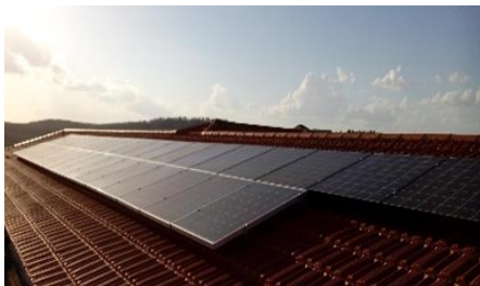
Figure 3: University of Évora's PV installation.
