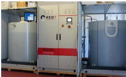
Figure 1: VRFB by manufacturer REDT, 60/5 kWh/kW, installed in the University of Évora.
