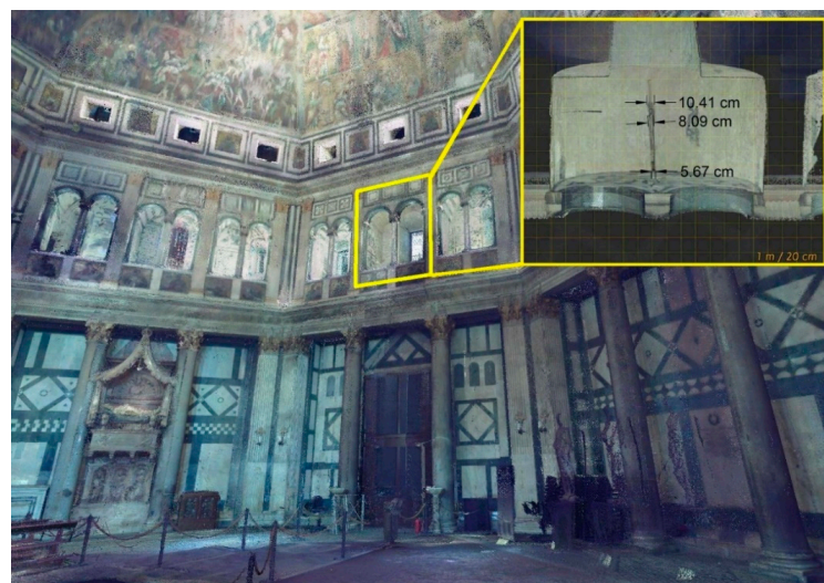
Figure 6. Scanning data highlighting the dimensions of a crack above the north door of the Baptistery di San Giovanni in Florence. Source: [29]. Figure 12, page 257.
