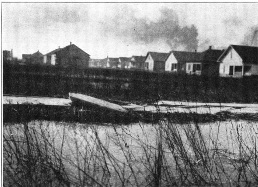
FIG. 17. BREAK IN SIDEWALK DUE TO SUBSIDENCE.
