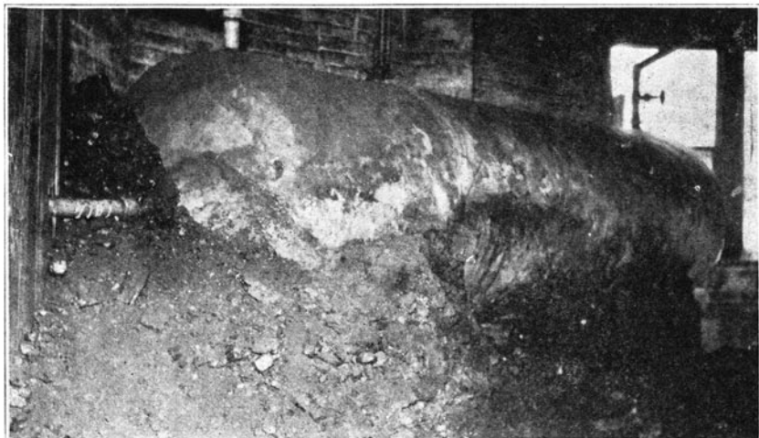
FIG. 16. COAL PILED AROUND HOT WATER TANK
