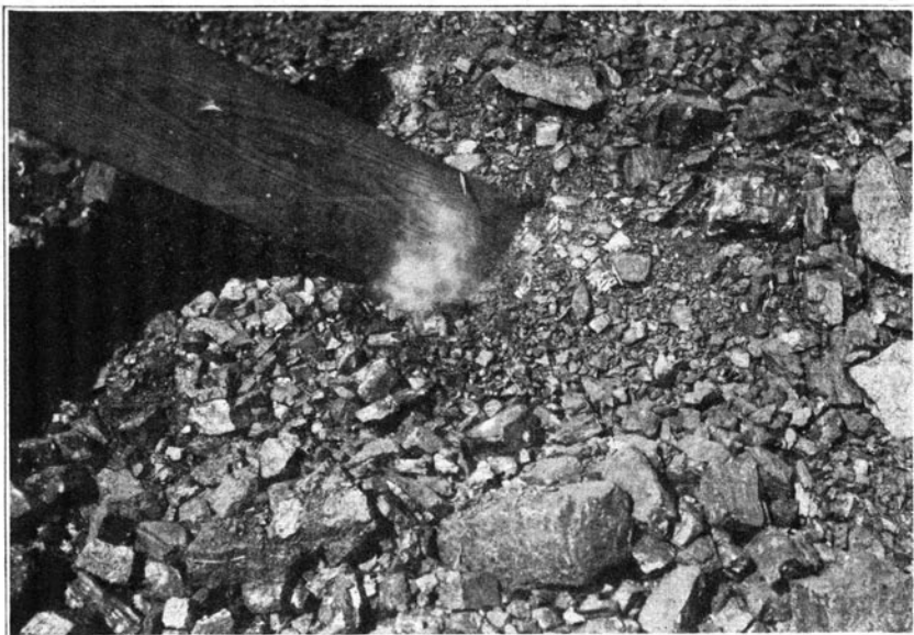
FIG. 23. FIRE STARTING IN COAL PILE AROUND EMBEDDED WOODEN BEAM
