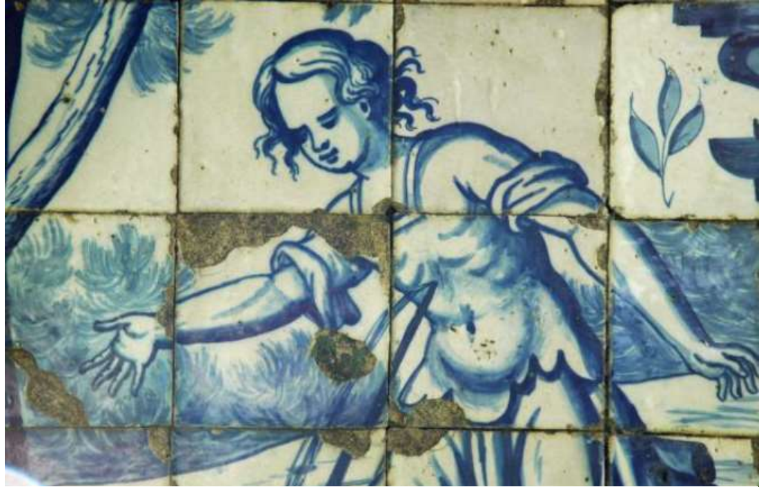
Loss of glaze and evidence of biological colonisation
