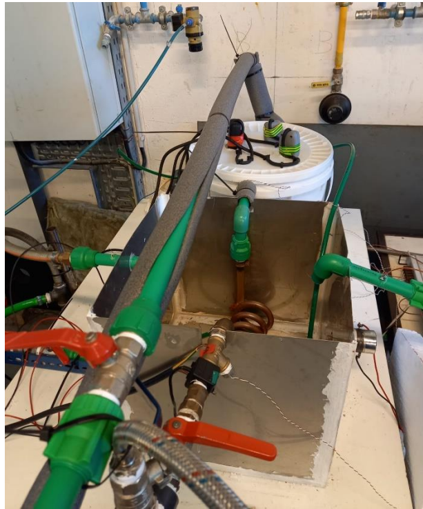
Figure 3.8 – Insulant applied in the hot fluid circuit.
