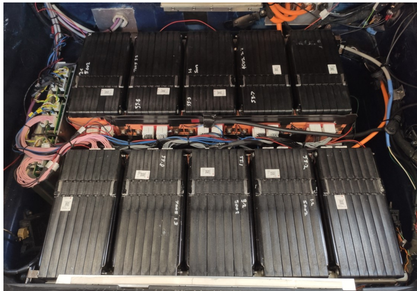
Figure 3.5: Pack of batteries installed in the back of the vehicle
