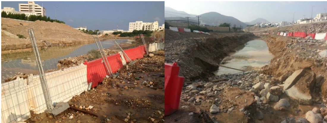
Fig.18 – Wadi four days after the significant rain event after the start of work
