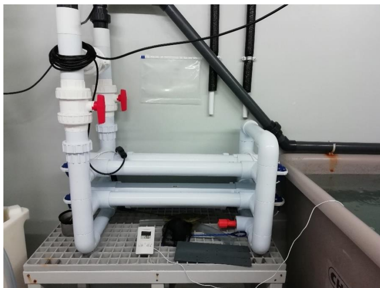
Figure 18 - UV disinfection lights used in BOGA.
