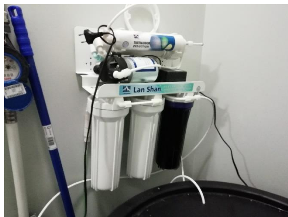
Figure 5 - Reverse osmosis system in BOGA.
