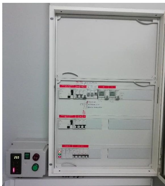
Figure 36 - Challenge room hall electric board and reservoir capacity display monitor.
