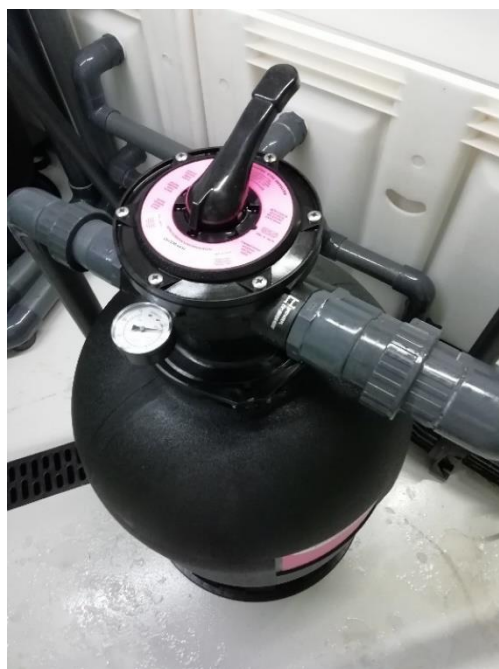
Figure 16 - Sand filter in stocking room p.09.
