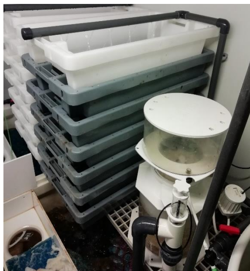
Figure 29 - RAS components in room p.09 sump – biofilters; protein skimmer; mechanical filters.
