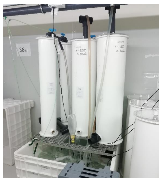
Figure 23 - Saltwater biofilter activation system 1.
