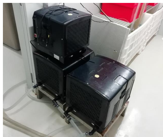
Figure 21 - Water coolers used in BOGA.
