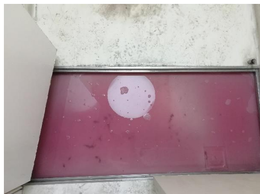
Figure 8 - Worn out footbath with accumulated debris.
