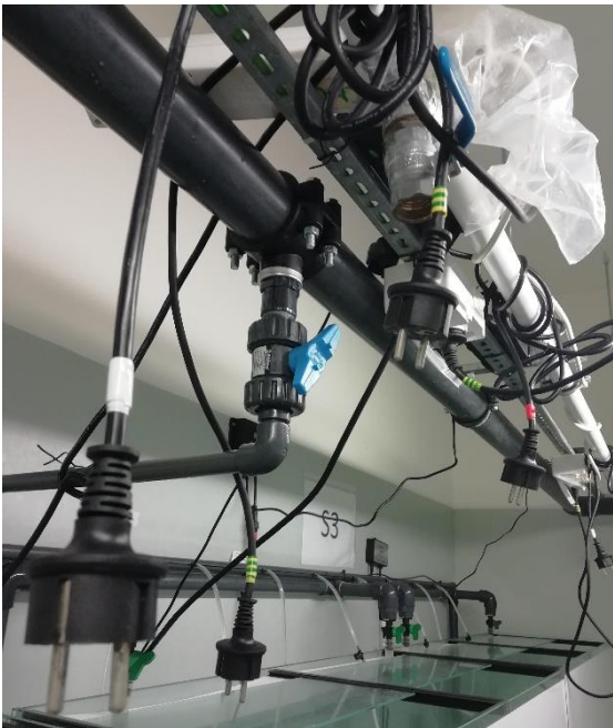
Figure 40 - Electric plugs in challenge room p.14.
