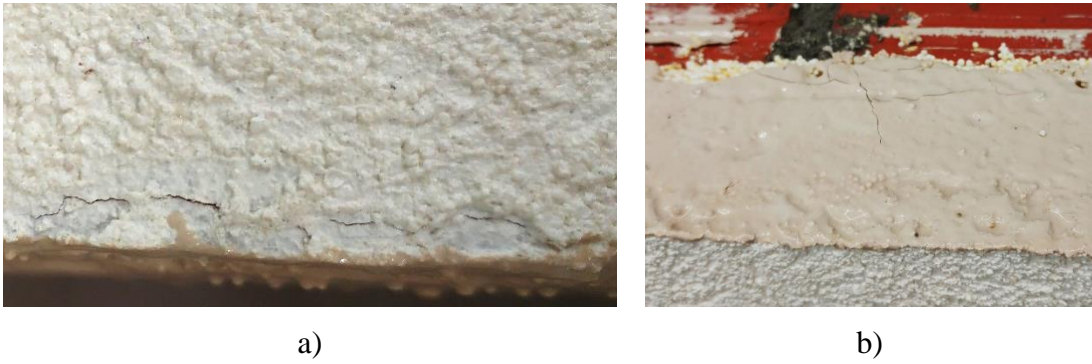
SM7. Representative damages: a) Damage of the coating; b) Cracks on the sealant, after freeze-thaw ageing cycles.
