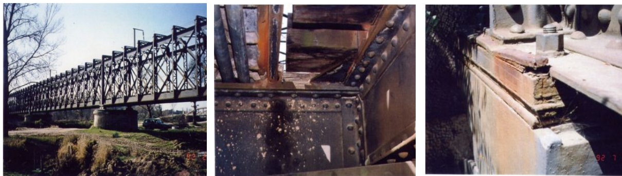
Figure 2.9 - Deterioration of the connections and corrosion of the metal elements in Soure bridge (Appleton, 2005).
