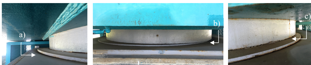
Figure 3.18 - Information obtained from visual inspections carried out on the bearings of piers P2 and P3 of the bridge over the Sado River.
