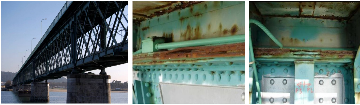
Figure 2.8 - Observed corrosion on the top flange of Eiffel bridge, Viana do Castelo (Cavadas, 2008).
