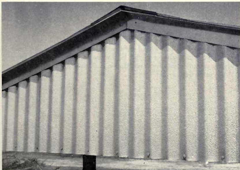
End section formed by riveting flashing or fastening with sheet metal screws. (Fig. 12)
