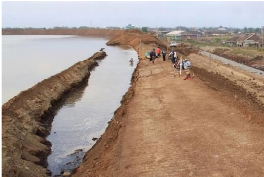
Figure 11 Internal erosion on 5 October 2018 is at around 150 to 250 m distance from P75A [46]. This means internal erosion caused by seepage.
