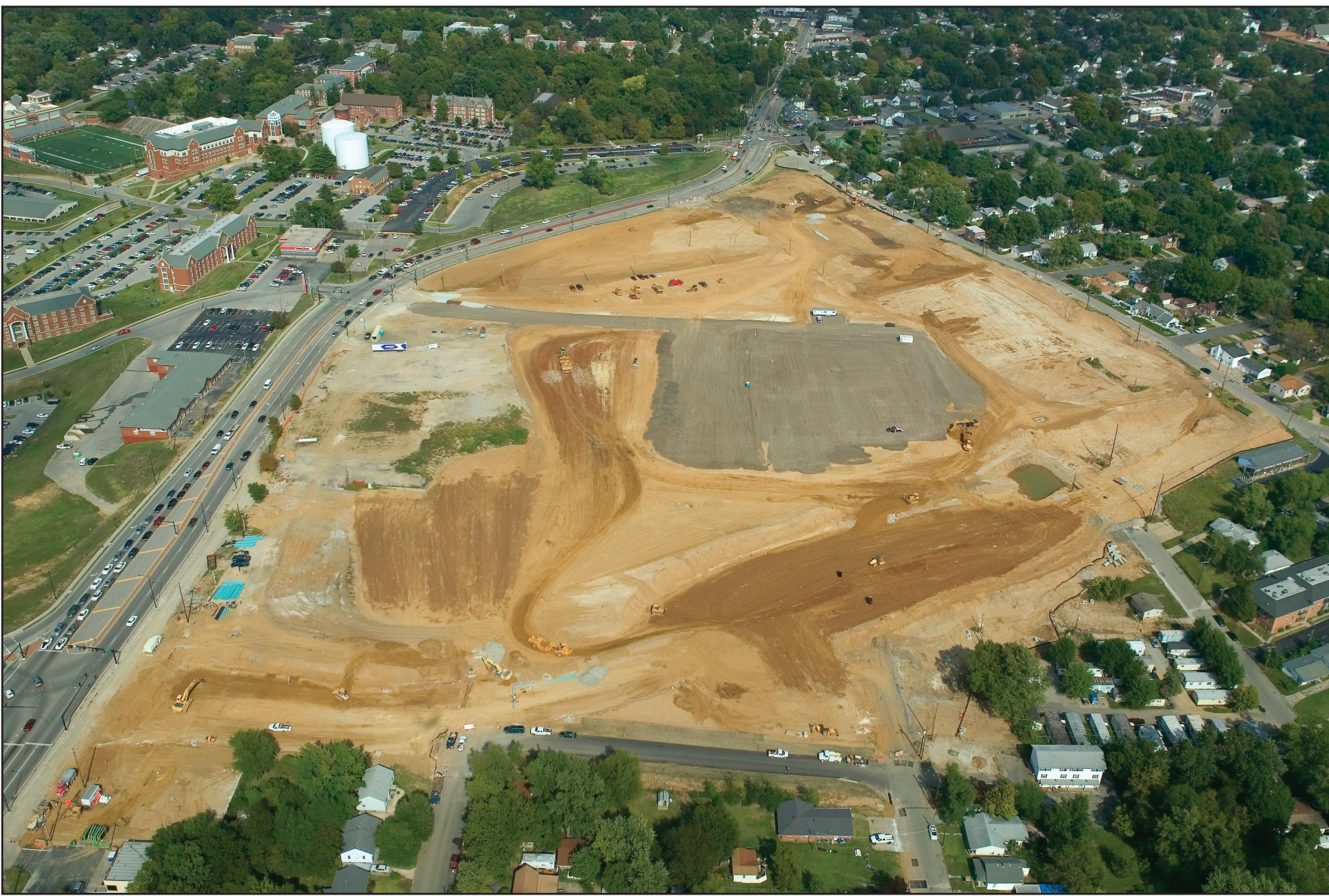
An aerial view of the construction site of the LU Commons across from Lindenwood University's campus. Photo Courtesy of DESCO Group
