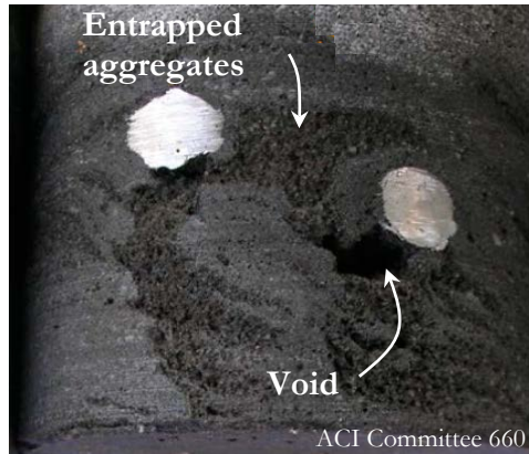
Figure 1.5: Imperfections created behind reinforcing bars (adapted from [30])
