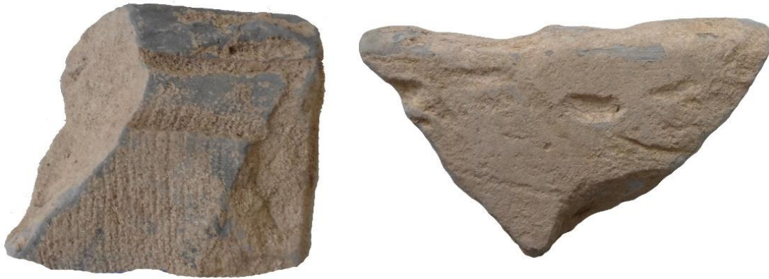
Figure 59 The horizontal traces on the concave surface of the roof tiles (Source: Photos by the author)
