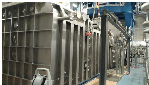
Fig. 6: View of the BLV installed inside MITICA bunker. The leak test of BSV+BLV (part of the SAT) was completed before the coronavirus lockdown.
