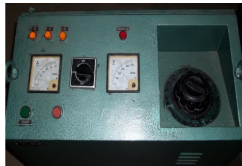
Fig 8. Wind Tunnel Motor Starting Equipment
