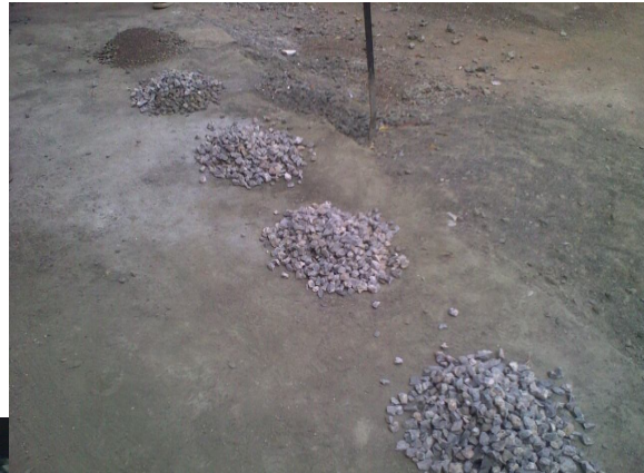
Figure 6 Batching of Cement Sand and Aggregates before the mixing and filling process
