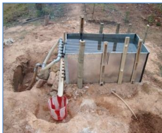
Fig. 6 : Testing of Condenser in Shillong.
