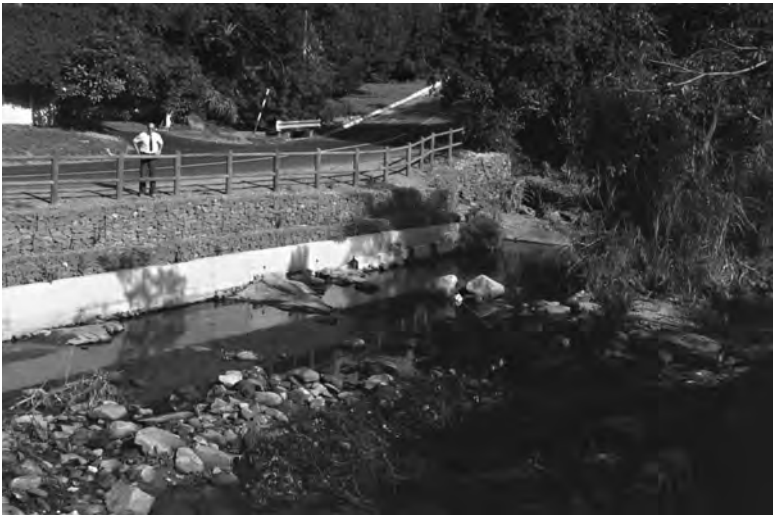
Photo 2: Gabions on a concrete foundation. Vegetation such as creepers could be used to soften the visual impact
