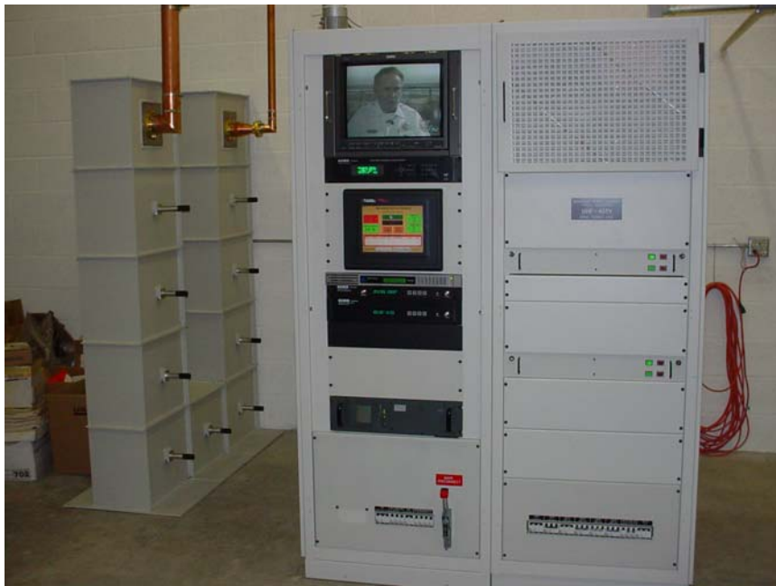
Figure 4.18 UHF-4DTV Transmitter Installed for KTFL Television in Flagstaff, Arizona.
