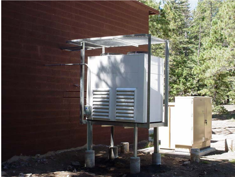
Figure 3.57 Refrigerated Chiller Installed at KTFL-TV in Flagstaff, Arizona
