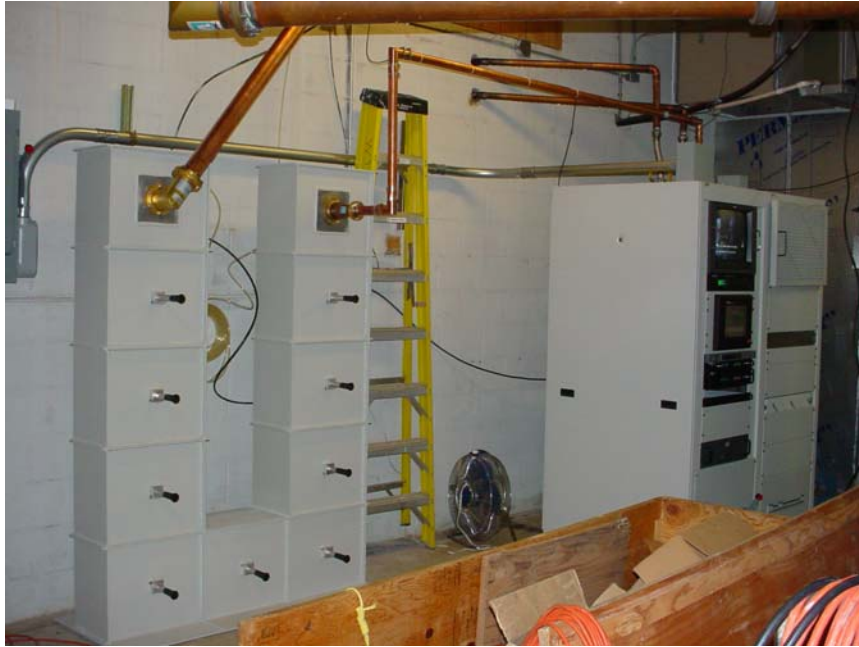
Figure 4.17 UHF-4DTV Transmitter Installed for WLOV Television in West Point, Mississippi
