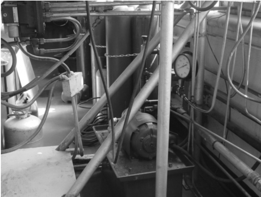
Figure C.3 Hydraulic Pump and Reservoir
