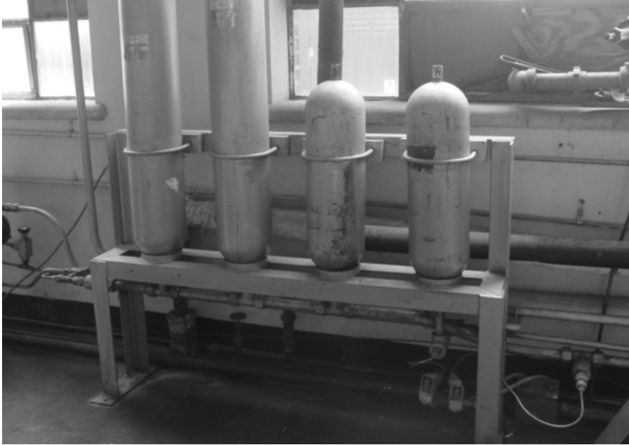
Figure C.4 Hydraulic Accumulators with Pressure Switches Below
