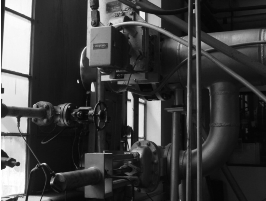
Figure C.6 Emergency Gate Release Valve with Inlet Butterfly Valve Above
