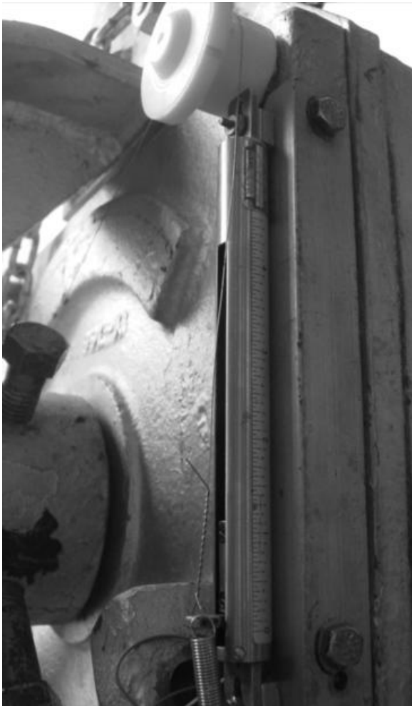
Figure 8 Potentiometer Used to Measure Valve Position
