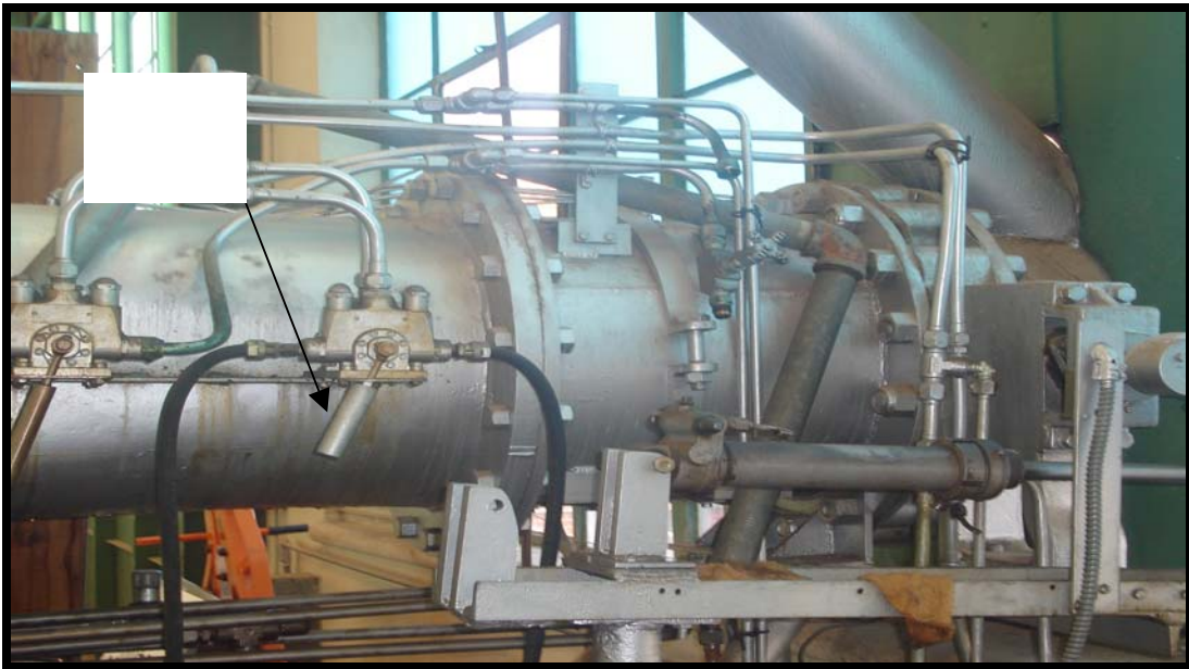
Figure 2.4 Downstream Valve Control Mechanism.
