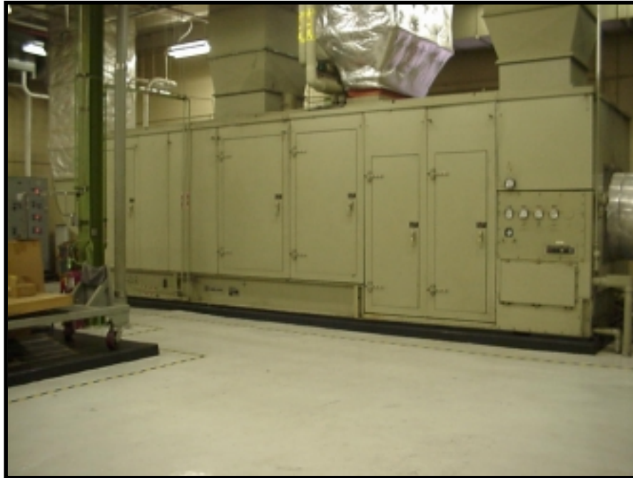
Figure 9.3: Centaur H Turbine Installation
