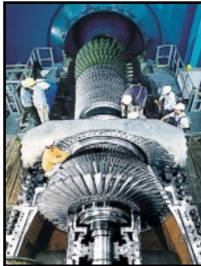
Figure 4.13: 157-MW Gas Turbine by Siemens Westinghouse ( www.siemenswestinghouse.com )
