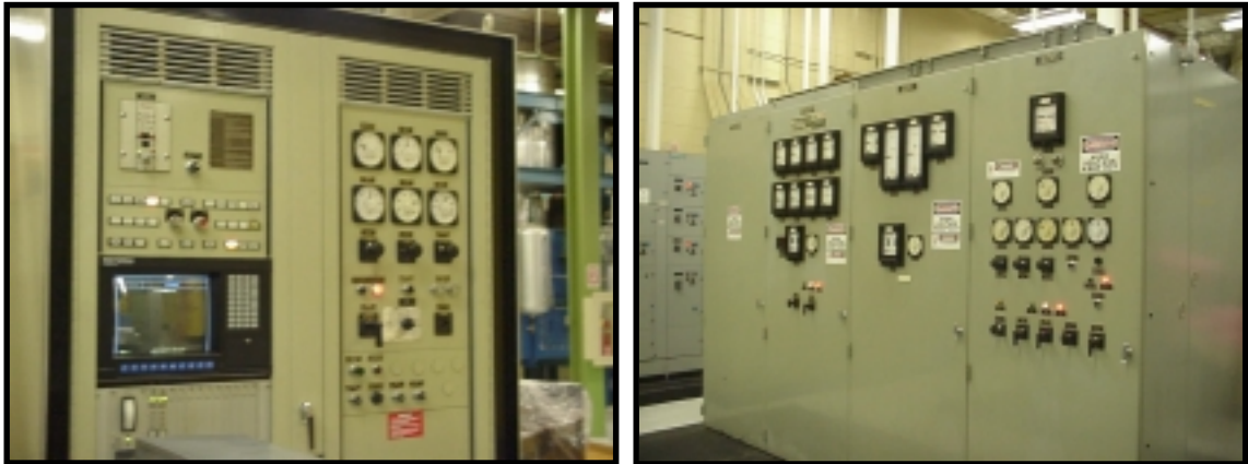
(a) Turbine Control Panel
