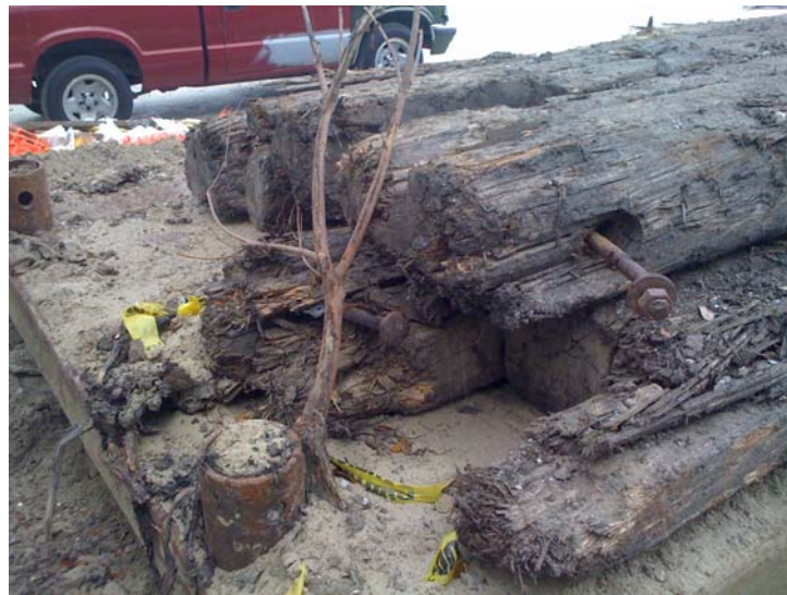
Figure 1.2 Damaged Wood Construction Platforms
