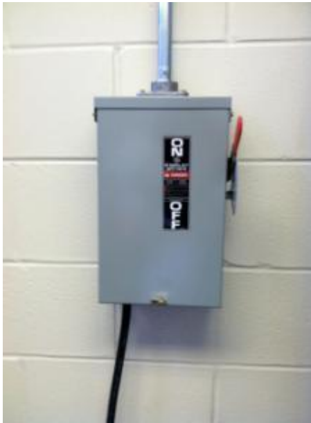
Figure C.1 Main power source switch.
