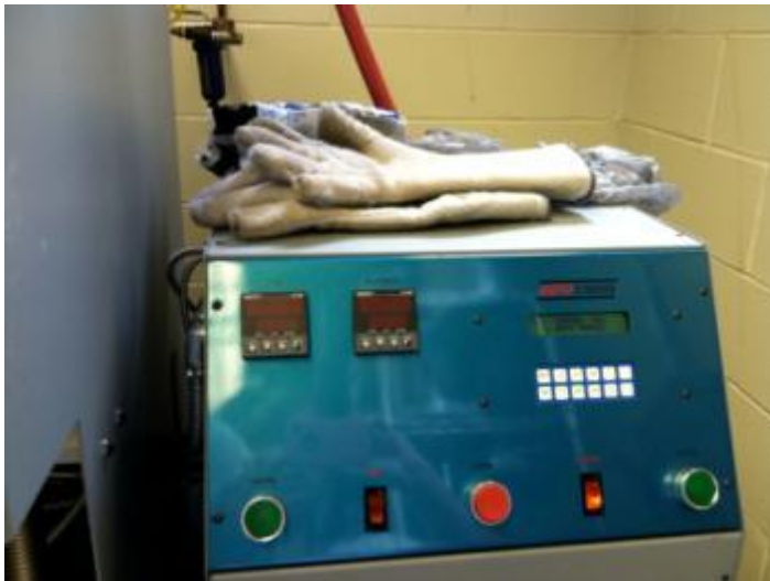
Figure C.3 Instrument control panel.
