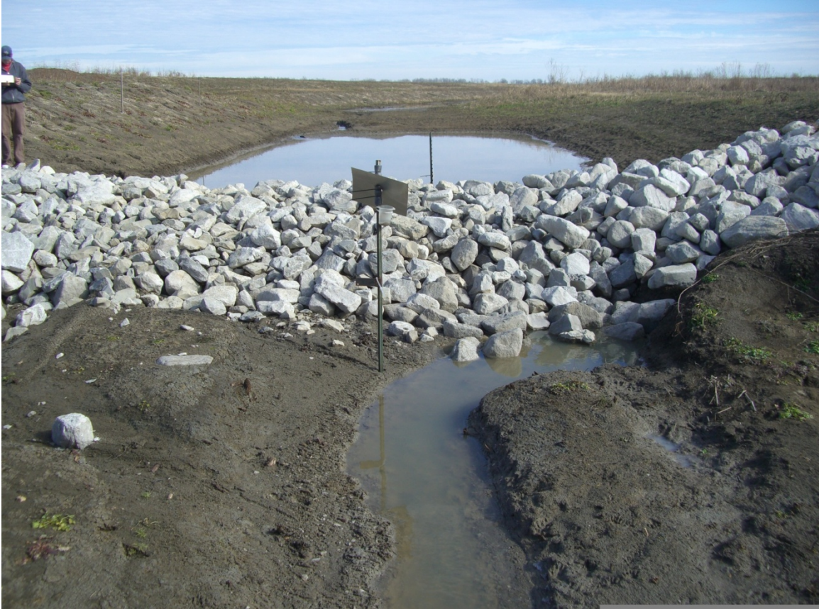
Figure 4.5 Photograph of Terrace Ditch, Yazoo County, MS, one month following construction in November 2009 and shows the upstream channel bed above the lower weir, revealing the ditch's lack of vegetation and bare soil.
