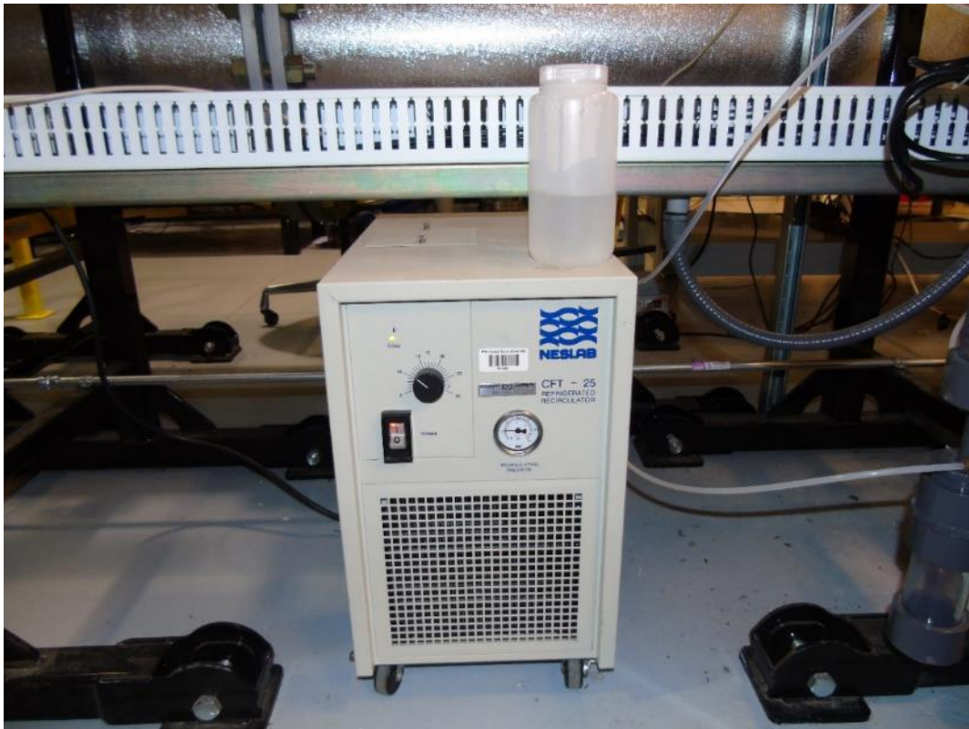
Figure 2.10 Chiller unit of the heat exchanger stages.
