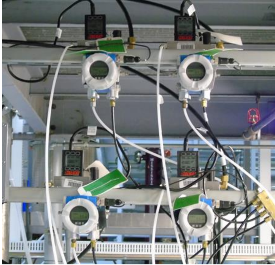
Figure 2.6 Mass flow controller and dP gauge arrangements for each sampler.
