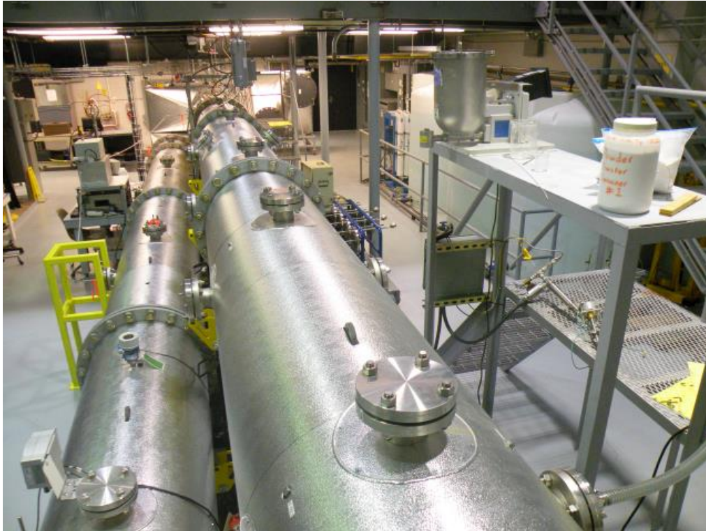
Figure 2.22 Configuration of the RLSTS with the isokinetic duct section installed.
