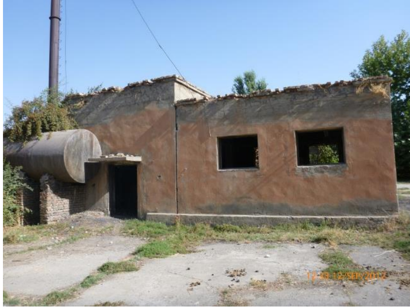
Figure C.11 Building housing secondary school heating system, in disrepair
