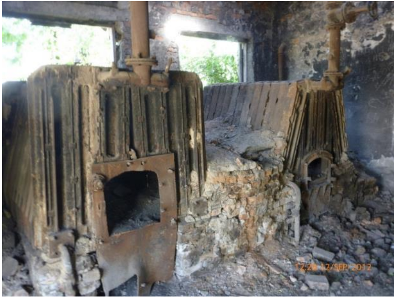
Figure C.7 Secondary school Soviet heating system in disrepair
