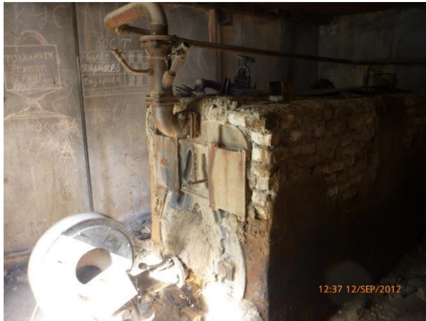
Figure C.13 Primary school Soviet heating system in disrepair
