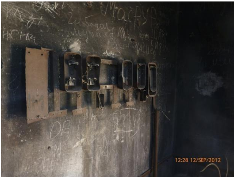
Figure C.8 Secondary school Soviet heating system dysfunctional
