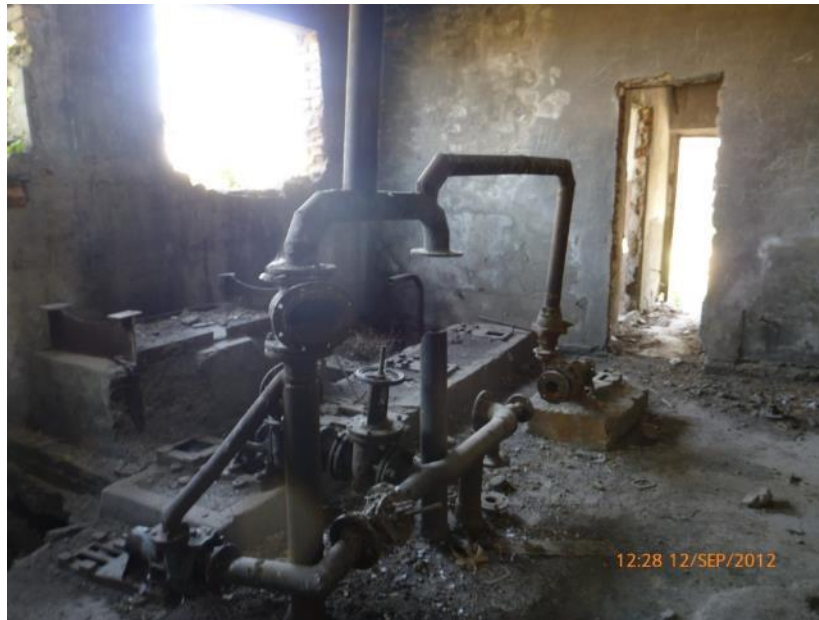
Figure C.9 Secondary school Soviet heating system broken
