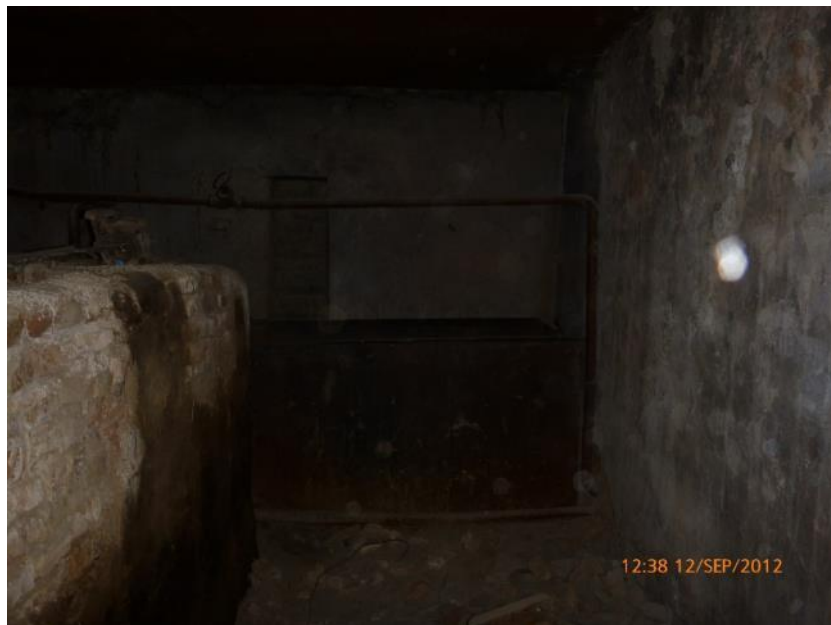
Figure C.14 Primary school Soviet heating system in disrepair
