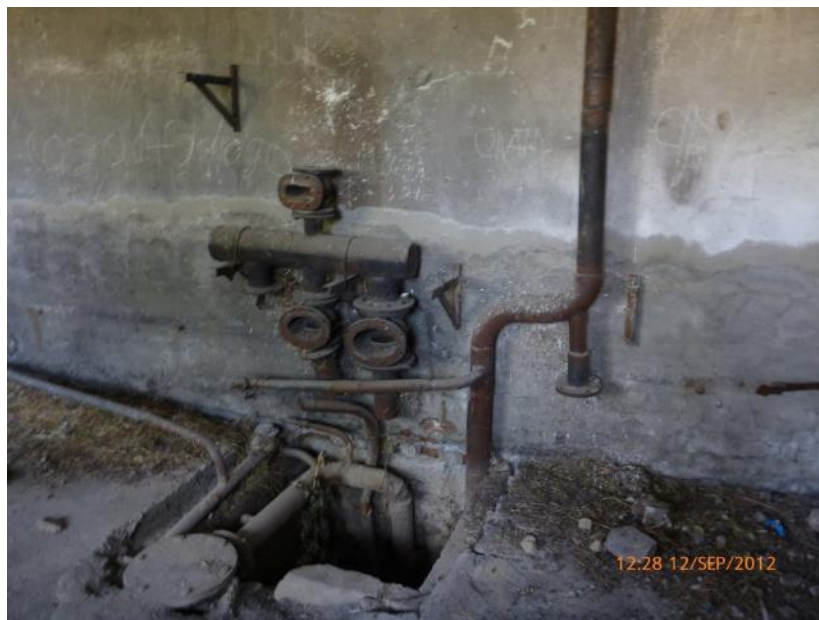
Figure C.10 Secondary school Soviet heating system broken
