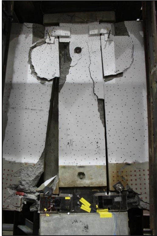
Figure 4.9 Elevation view, posttest condition of the center column/stud
