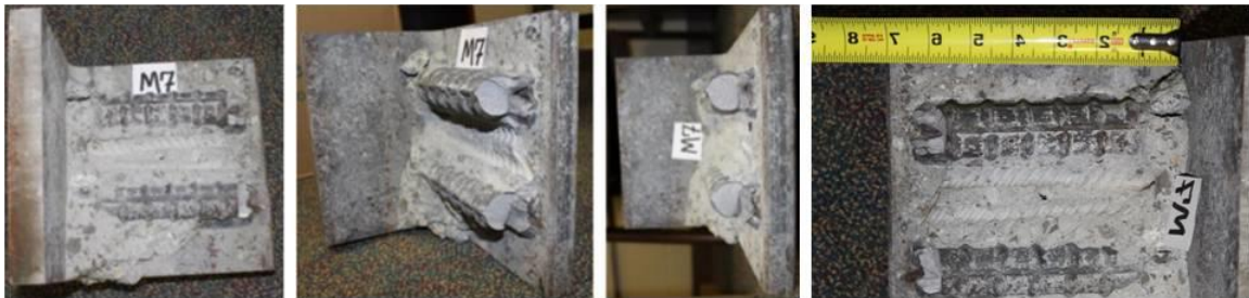
Figure 5.11 Different angles showing the location of fracture of the M7 anchor bars embedded in Beam-L near the center column
