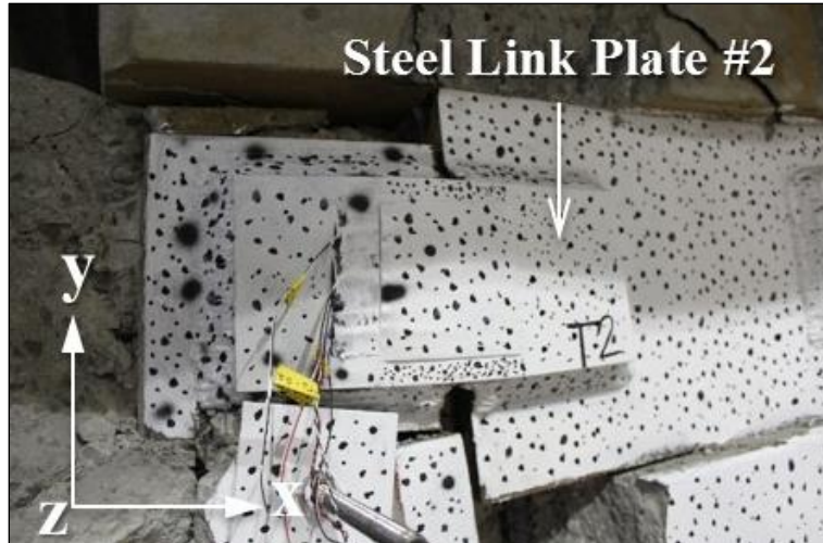
Figure 5.26 Close up view to posttest damage steel link plate #2
