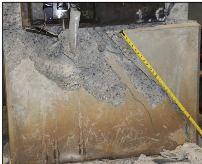
Figure 4.11 Elevation view, posttest damage of bottom of the right (west) end-column
