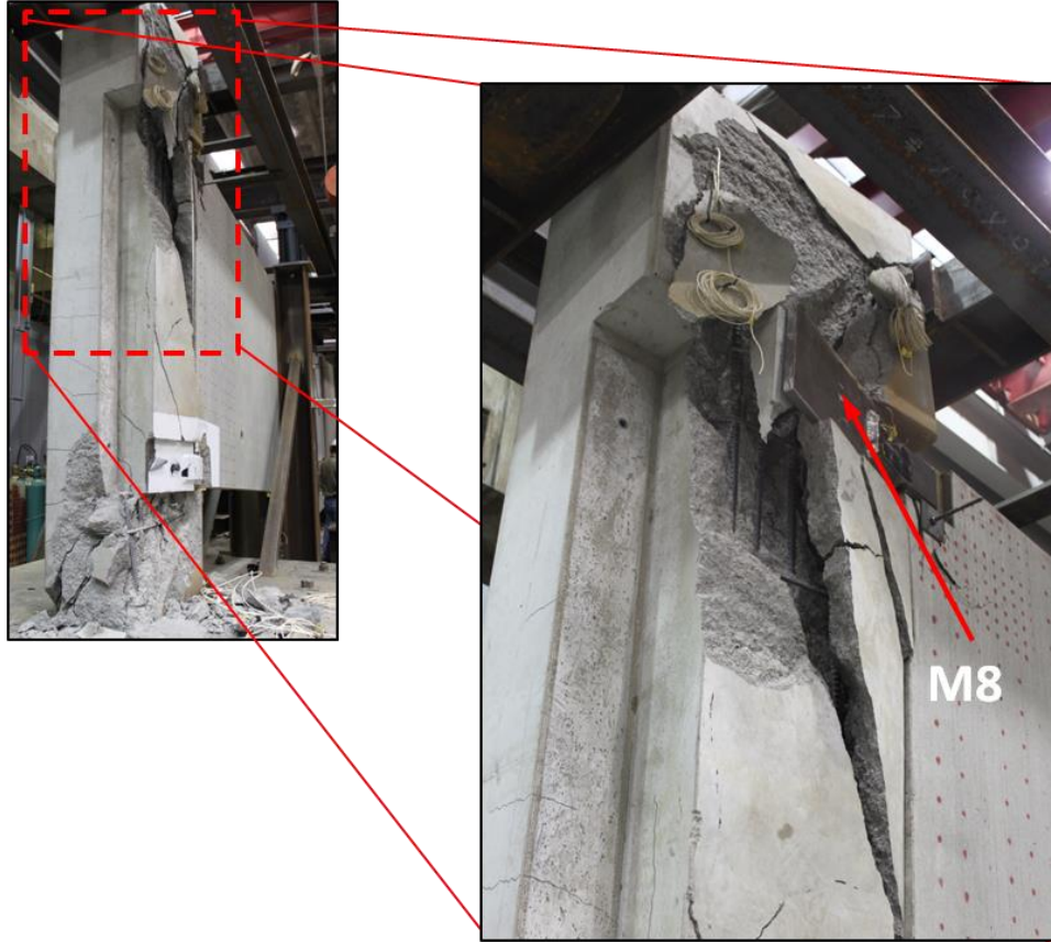
Figure 4.8 Elevation views, detachment of the upper M8 plate in the left (east) end-column
