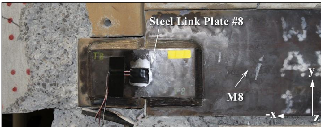
Figure 5.32 Close up view to posttest damage steel link plate #8
