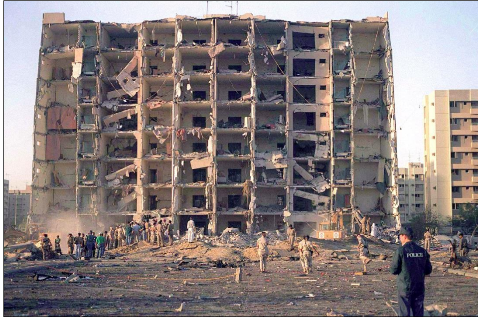
Figure 1.3 Side of Khobar building facing the explosive (KTBD, 1996)
