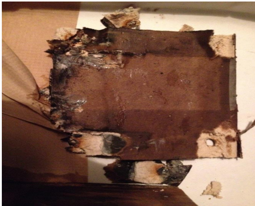
Figure 3.11 Picture of gypsum wallboard bottom brown paper (side facing the insulation) side on extraction day 65
