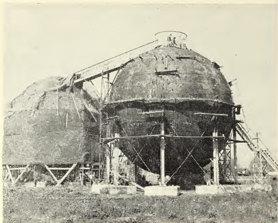
Figure 5. Two Horton spheres under construction. Each sphere has a capacity of 210,000 gallons. The pressure in Horton spheres is usually maintained at 60 pounds per square inch or less by means of refrigeration.
