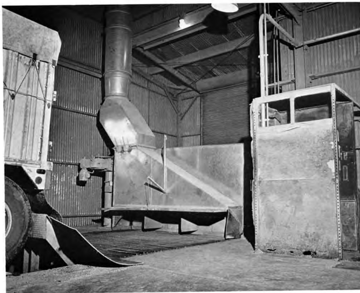
Figure 11. Dust hood installation for unloading pit. Hood is swung to in-use position.
