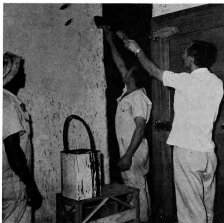
Figure 1. Foil-laminated vaporseal applied with asphalt compound to eliminate danger of moisture entering seed storage room when cracks develop.
