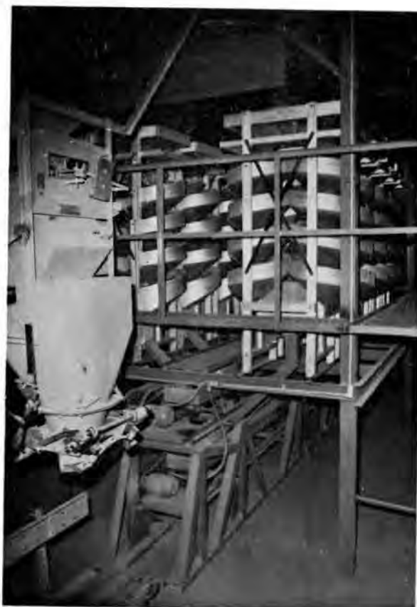
Figure 1. Spiral Separator installation in a Wilson, Arkansas, Soybean Processing Plant.
