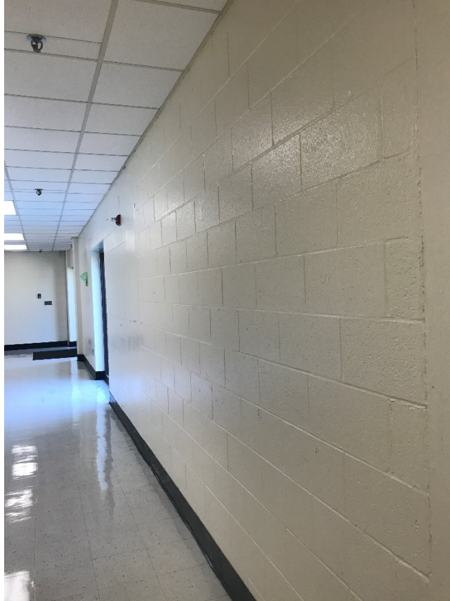
Structure 43 is a One Hallway Addition to Structure 42 Concrete Column Exposed
