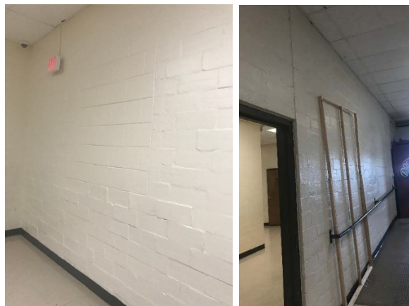
Interior, Damage to Masonry
