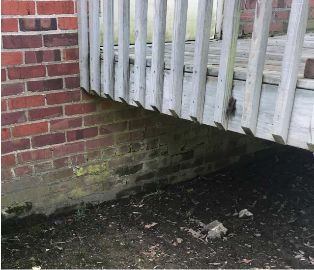
Exterior, Cripple Wall
