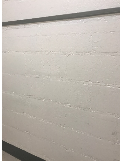
Masonry, Visibly Aged
