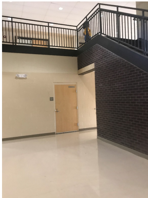
Joint Between Structure 42 (White Façade into Page) and Structure 44 (Stairs Out of Page)
