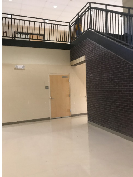
Joint Between Structure 42 (White Façade into Page) and Structure 44 (Stairs Out of Page)
