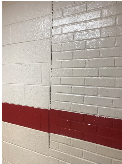
Connection Between this Portion (Left) and Older Portion, Visible Cracking
