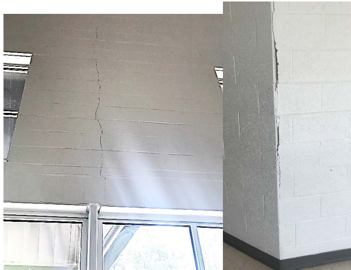
Cracks in Structure, Evidence of Pounding and Deterioration/Settling
