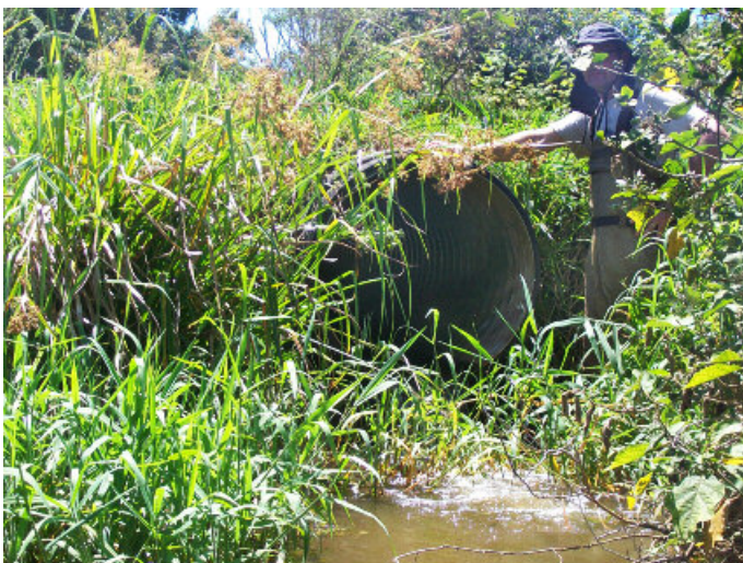
"Barrier" formed by the lower causway on Williams Creek East Branch.
